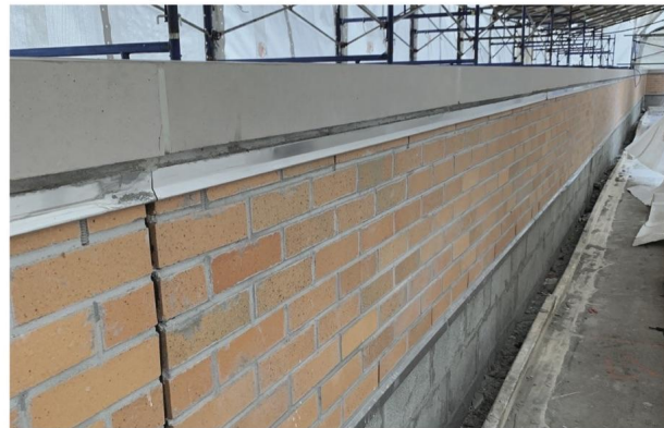
► With the copings and flashing in place, the parapet is nearly complete.
