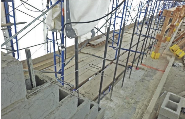
► Steel bars reinforce the concrete masonry unit core of the new parapet.
